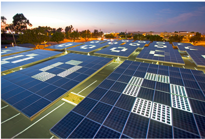
A "solar grove" built by Envision Solar for Kyocera's offices in San Diego. (Credit: Envision Solar)
